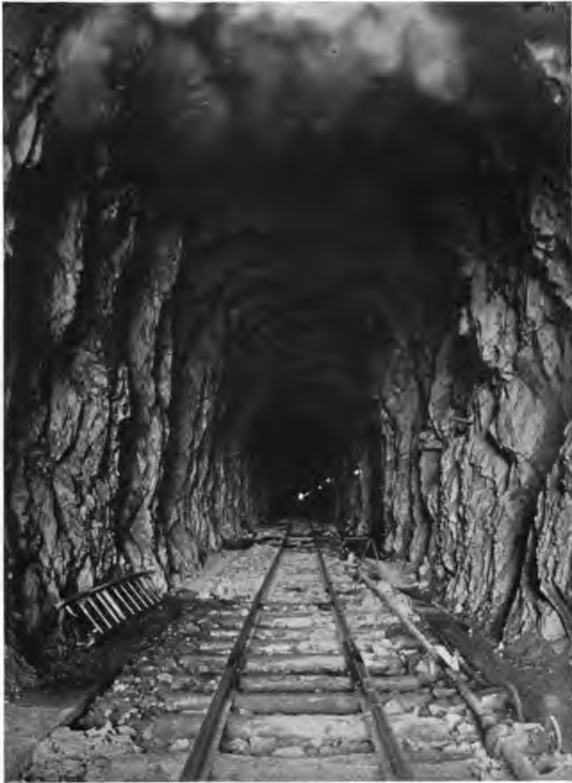
PLATE 77. —Peak Tunnel Fully Excavated and Ready for Concrete Lining. Footing Courses are in Place. Center Track for Hauling Material, to Upper Portion of Contract 11. Tunnel is 3450 feet long on tangent.
